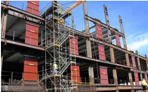
113 VWDs were installed in the $1.6 billion Geary Van Ness Medical Center project in San Francisco, California.
