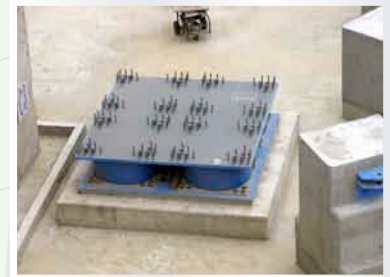
Groups of four isolators are located under heavily-loaded columns in the Tan Tzu Medical Center.
