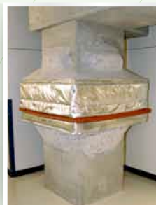
Fire blankets were used in Channing House.
