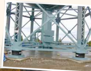
Retrofitted water tank in Seattle, Washington.
