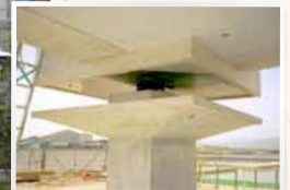
Top: Yuzawa Hospital, Japan. Bottom: A slider installed at Takasu Hospital, Japan.
