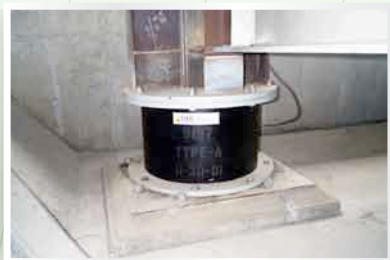
Isolators in the Long Beach 911 Center required no fire protection.
