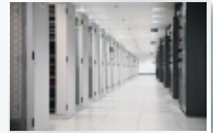
A DIS Low Mass Isolation System can be used to isolate a whole floor or an individual server.
